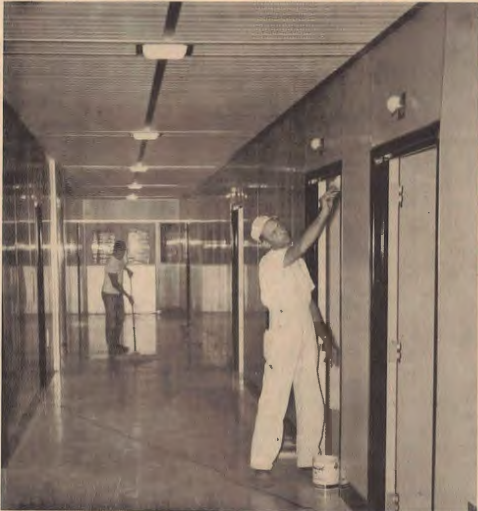
THIS is a picture of remodeling activities on one of the halls of the original building at Arkansas Baptist Hospital.
