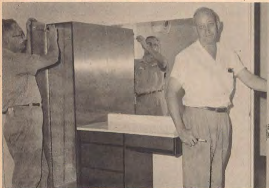
Installing the combination closet and vanity in one of the remodeled rooms is Ed Michell of the Maintenance Department while Chief Engineer Sid Coryell opens one of the new doors.
