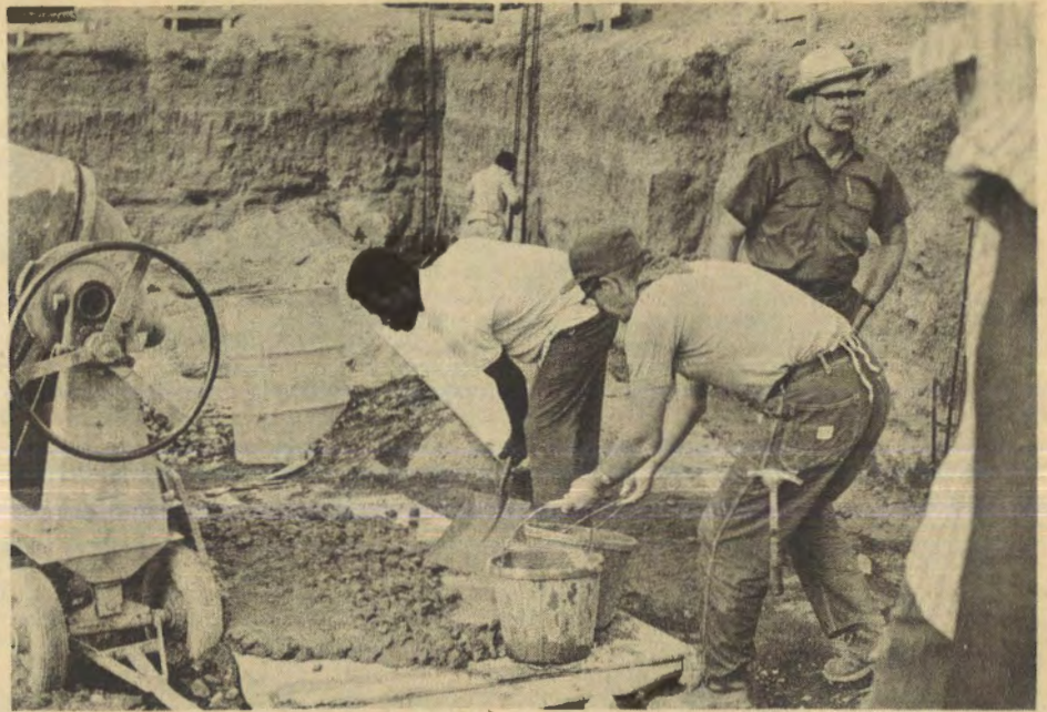
CHURCH CONSTRUCTION IN WEST INDIES: Illinois Baptists work with a member of Mt. Carmel Baptist Church, St. Kitts Island, West Indies. The men are carrying concrete to pour footings for a new church building on the island. Nine Baptist men from Illinois worked two weeks, helping local Baptists construct the new building, which will serve several villages. (BP) Photo by John Whitman
