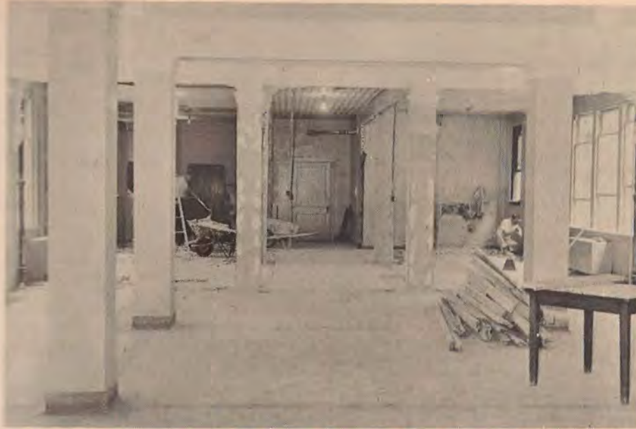
This is the way the chapel now looks with the back wall removed. The new laboratory will be built in this second floor section of the hospital.
