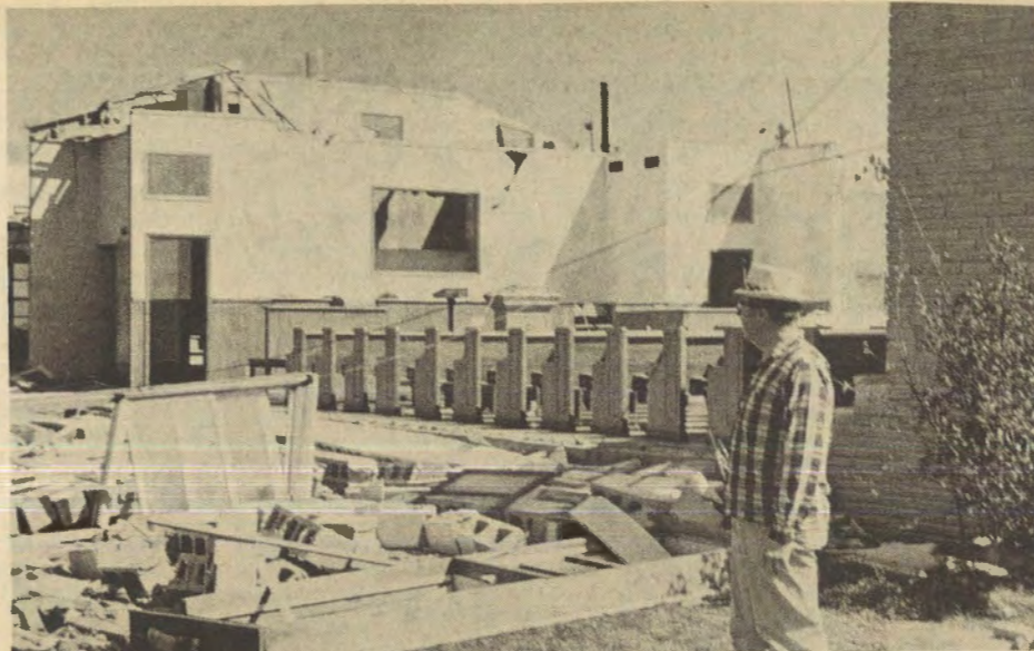
TORNADO DEVASTATES CHURCH: Pastor Leon Piper surveys the ruins of Highland Park Church in Conyers, Ga., after a tornado destroyed the sanctuary and half of the education building. Although only partially covered by insurance, the church hopes to rebuild. (BP) Photo
