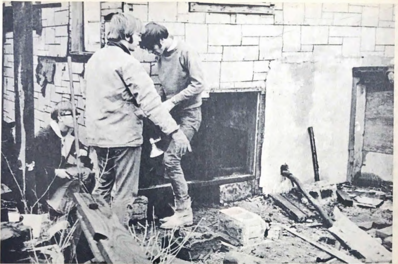
Repairs on a dilapidated building are begun by Richard Knight of U of A, Gomer Newton of Southern State, and Robert Tollison of UAM.
