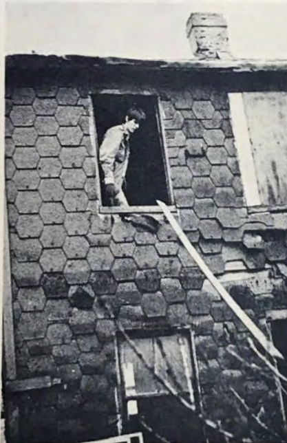
Jimmy Jones of Southern State pitches out a piece of lumber not needed in the repair work.
