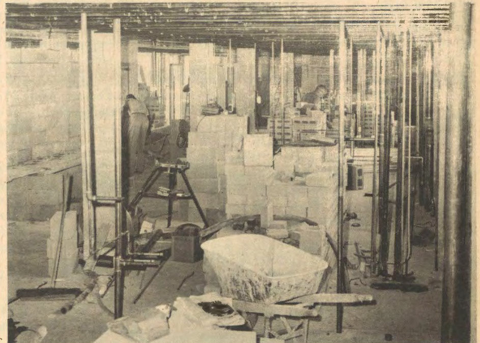
By the end of the year, the Hospital hopes to have pediatrics patients in this remodeled section of fifth floor. It is part of the extensive remodeling work being done on the entire east wing of the Hospital.
