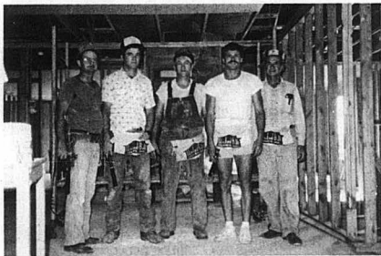
North Arkansas Association Brotherhood mission team was in Indiana July 18-25 to assist Oak Hill Church in Evansville with re-roofing its present sanctuary and completing its new educational building. Team members installing sheet rock and insulation to classroom walls were (left to right) Paul Dart, Glenn Sattler; Nolan Brisco, associational Brotherhood director; Tim Cooper; and Albert Thompson.
