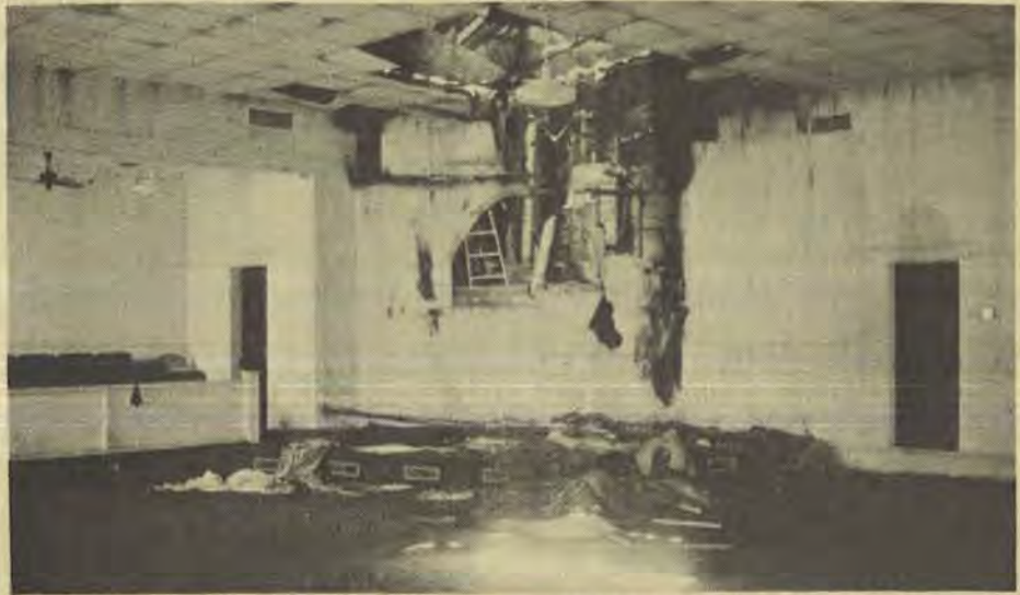
The fire in the building of First Church, Bearden, began in the baptistry (center) and burned through the roof. Parts of the building besides the immediate area suffered heavy smoke and water damage.
