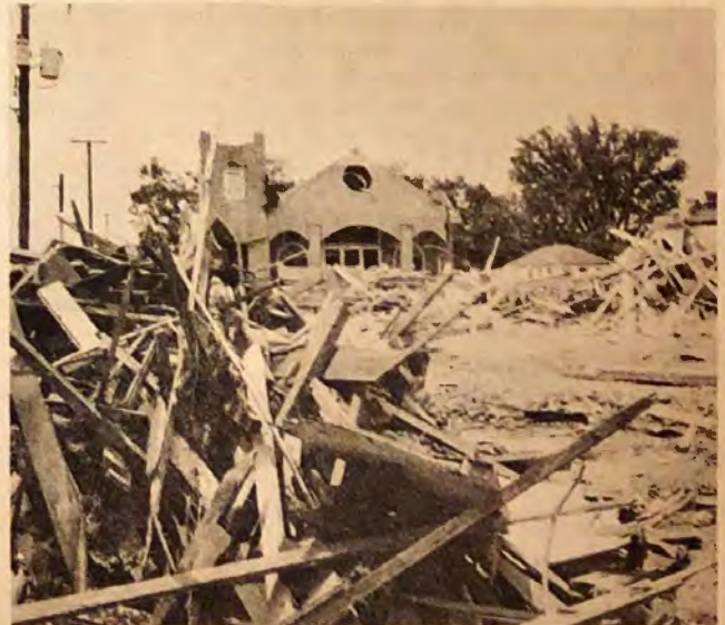
This black church received some heavy structural damage. All Southern Baptist churches escaped damage.
