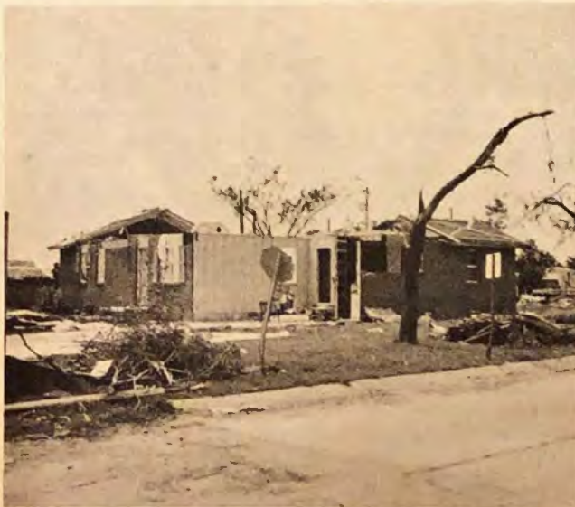
This home lost the roof. This middle class area suffered relatively light damage.
