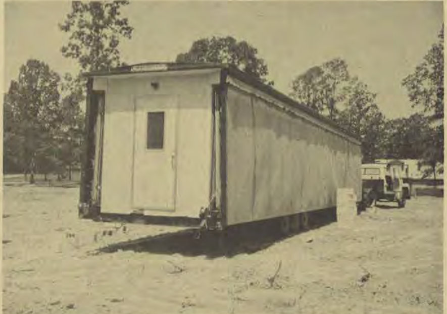
In late June the chapel arrived on the site of the new mission venture in Redfield, Harmony Association. It was ready at this point to be unfolded and leveled to provide a 24' x 53' building until the permanent one is erected.
