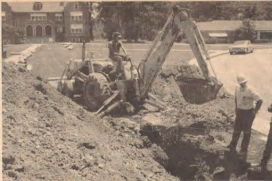
WORK AT CHILDREN'S HOME —Work is in progress on a new eight inch sewer main at the Arkansas Baptist Home for Children. This line replaces the original four inch main which was installed in the late 1920's. The cost of the project is $5,000. The original sewer system served four buildings, but the Home has grown now to include nine buildings.
