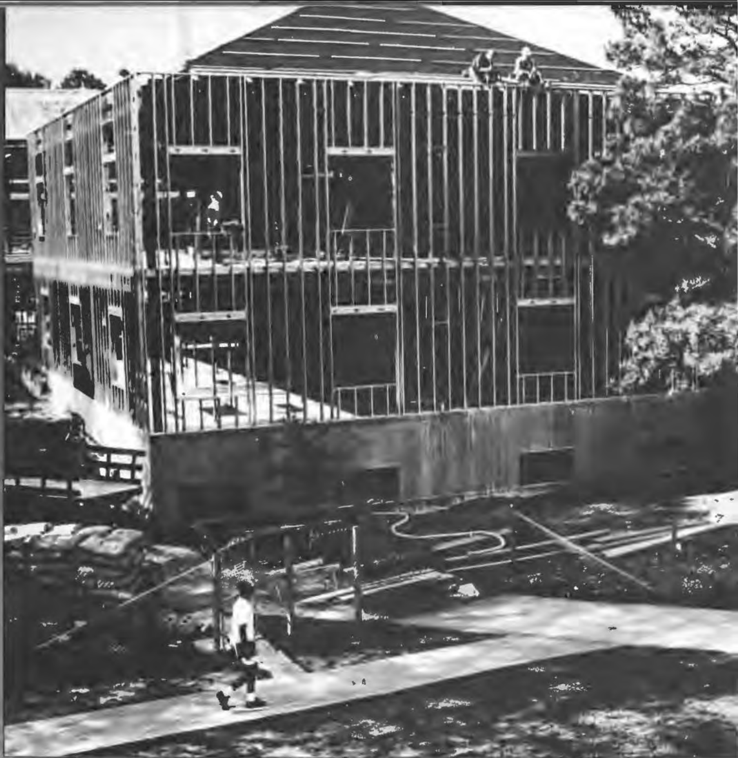
Going up. Workers from Pickens-Bond Construction build the frame to the new Riley-Hickingbotham Library. The facility was completed for student use in the fall.
