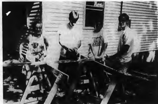
Twenty-two young people from Second Church of Little Rock assisted Aug. 8 with a Habitat for Humanity construction project at 4007 Ludwig in Little Rock. Building porch rails were (left to right) Eva Umboltz, Richard Binns, Reagan Binns, and Brad Williams. Youth Minister Paul Warren coordinated the volunteer effort.
