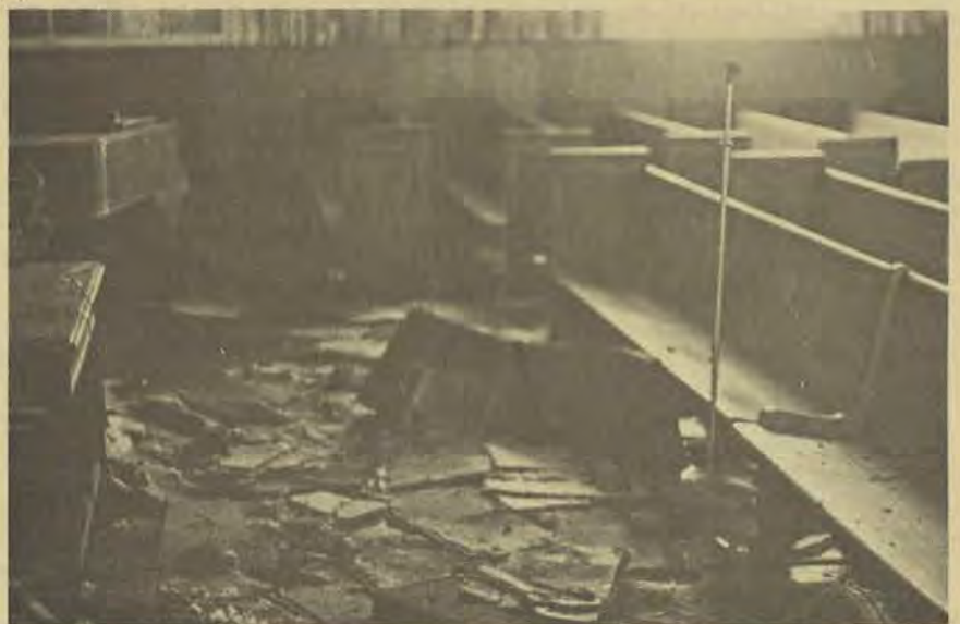
A fire Saturday, April 9, at South Highland Church, Little Rock, heavily damaged the sanctuary. The area most heavily damaged was above the pulpit area (top photo). Debris from the ceiling covers the floor and soot and water stains show on the walls. The bottom photo shows a closer view of debris from the burned out attic. Roy Cook is pastor of the church. (ABN photos)
