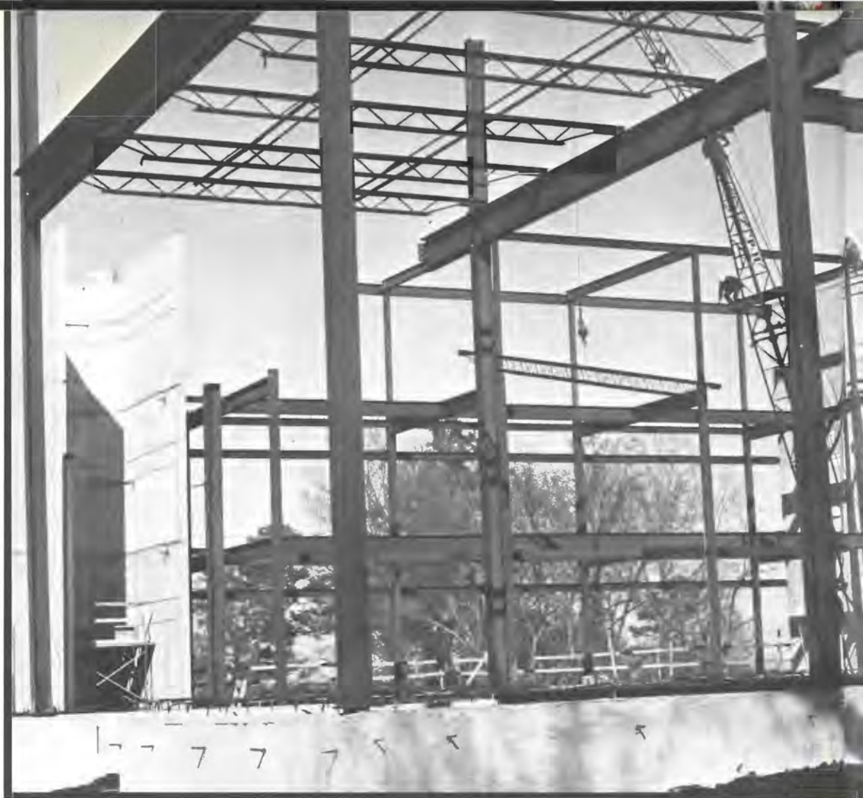
Fine Arts (Right) Building construction is kept on schedule for August completion.
