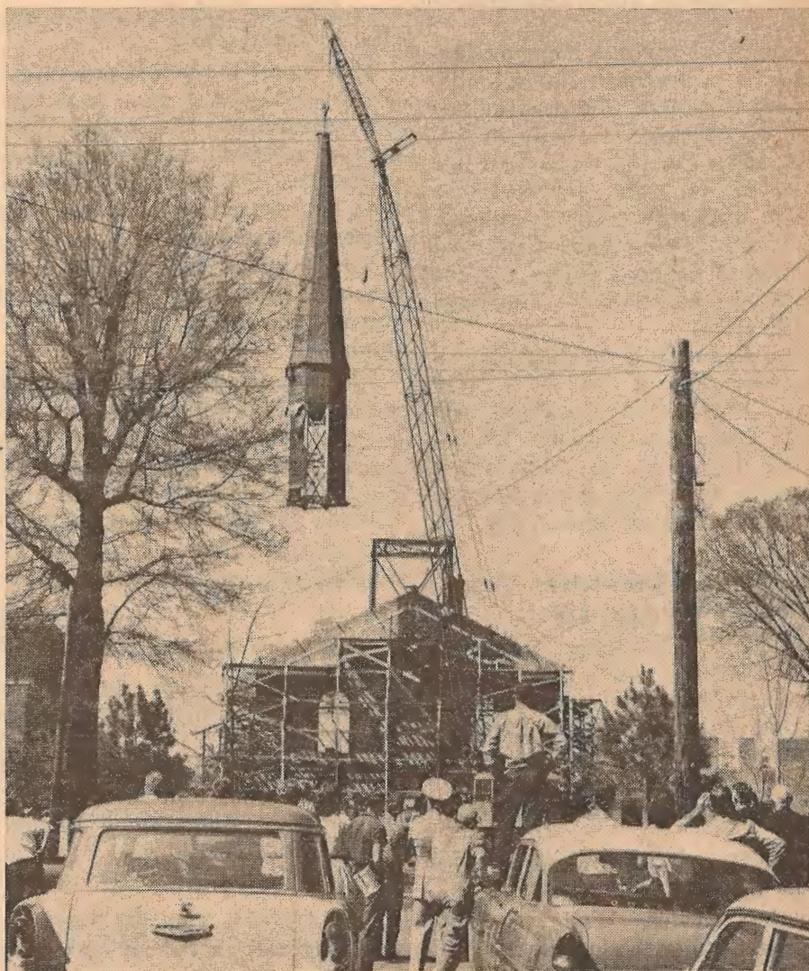
A HUGE sidewalk throng gathered April 13 to watch a crane from Arkansas Foundry Co. lift the tower for Ouachita College's $200,000 Bible Building, now under construction. The tower stands 104 feet high from ground level, the highest elevation in Arkadelphia. ■
