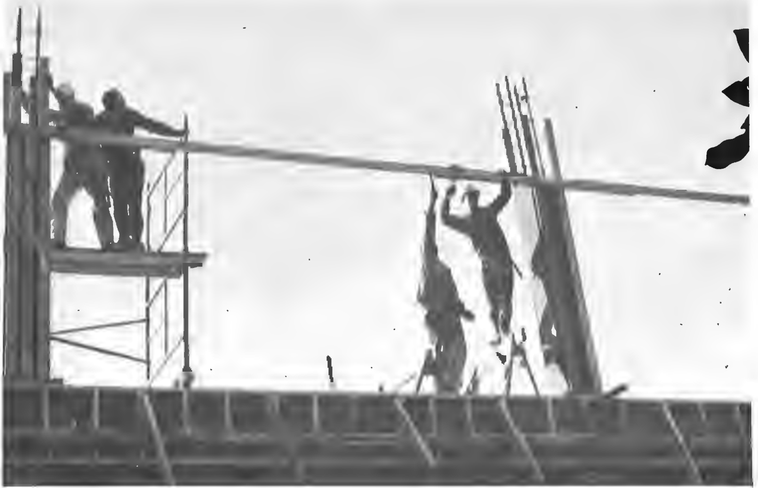
Lining up of wooden framework was the prelude to another floor as the addition to Riley Library went up.
