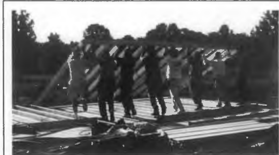
The Calvary Volunteers, a group of men from churches in Calvary Association, recently assisted in construction of a new sanctuary for Central Church of Bald Knob where Claude Gibbs is pastor. Larry Gray of Rocky Point Church served as construction supervisor.
