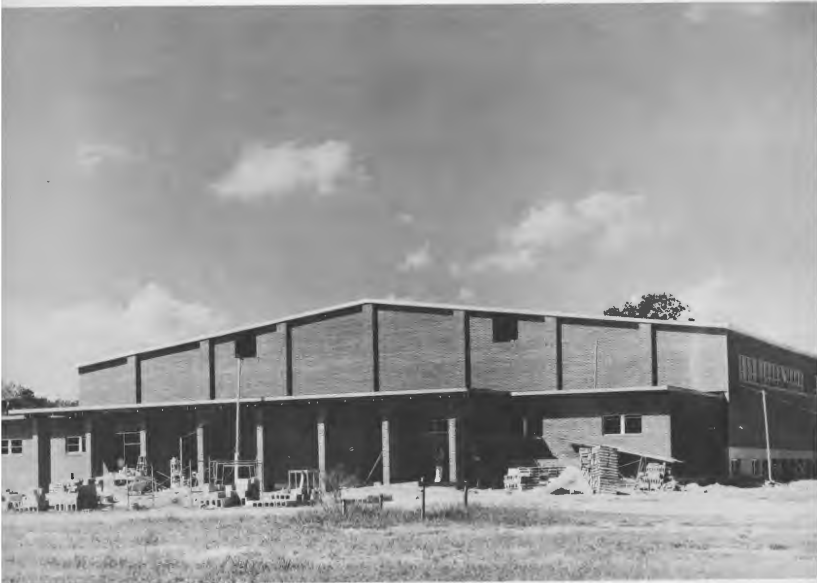
Even though lack of funds delayed construction, the new gymnasium was ready for the second basketball game of the season.
