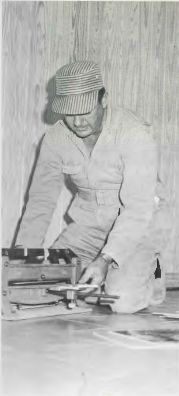
Trimming tile to fit the floor, the president pitches in to help so that the student center annex will be completed by Homecoming.
