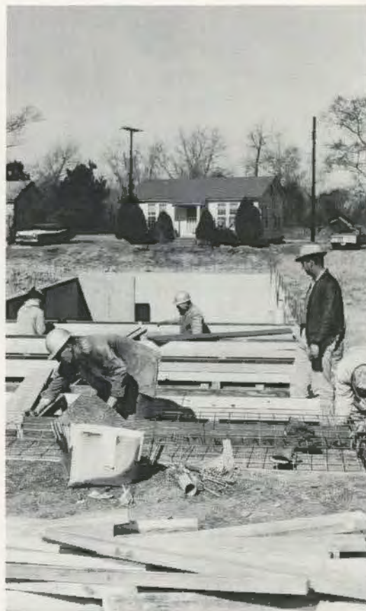
Construction of the new gym gets well under way with Gary Stephens, Leroy French, and other members of the campus crew doing the construction.
