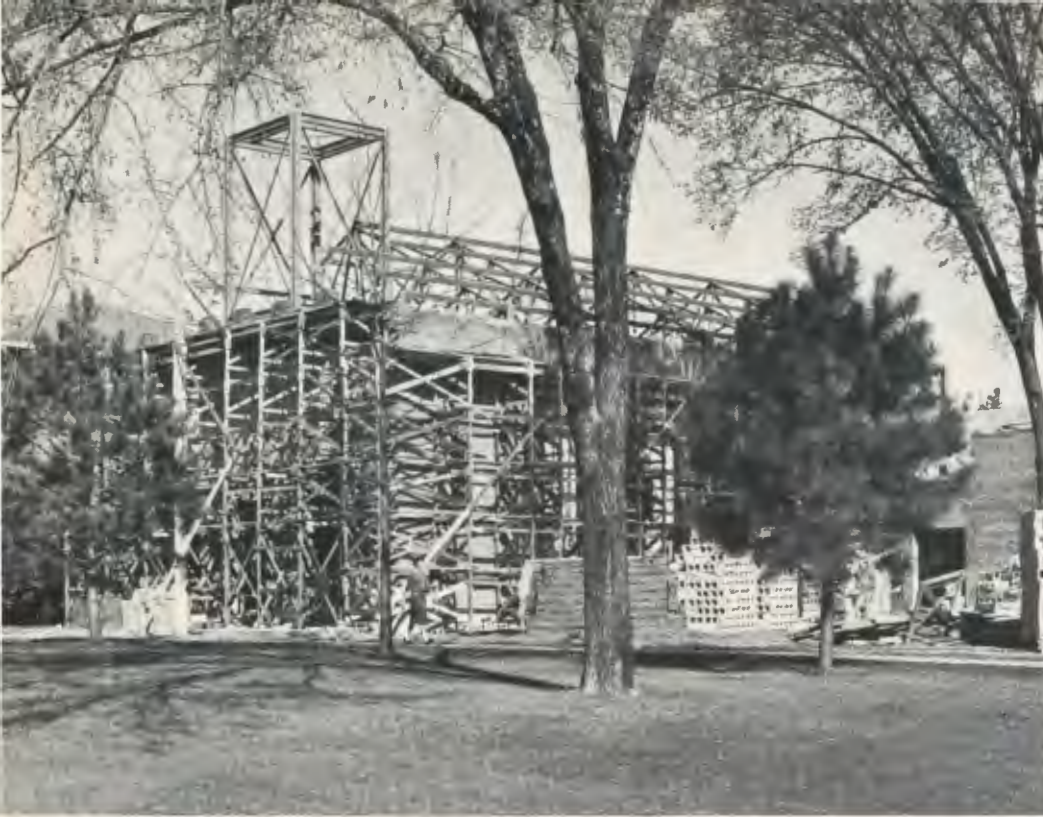
Construction for the new chapel, to be named after Mr. J. E. Berry, was speeded up as the weather grew warmer in the spring.
