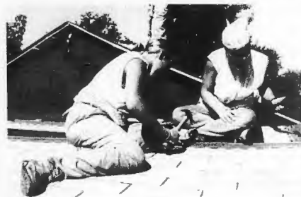
Most of the World Changers projects in West Memphis involved participating youth re-roofing homes and repairing porches.
