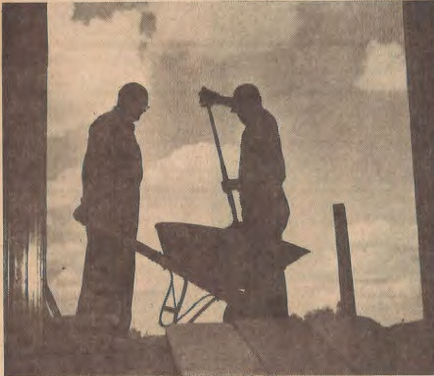
FORT WORTH—Men and shovels, silhouettes against the sky, continue to provide the basic labor needed for modern-day construction. These Southwestern Seminary students, employees of the seminary plant department, are among those working on Cowden Hall in a $500,000 "face-lifting" which will make this School of Church Music building one of the most modern and functional music buildings in the nation.
