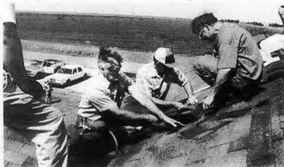
Larry Ballinger (left), a member of Highland Drive Church in Jonesboro, was part of the Mt. Zion Association construction crew that repaired the roof of Shiloh Church in Lake Village during a recent Mississippi River Ministry in Delta Association.
