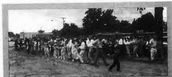
Members of First Church of Dumas "pulled together" June 29 to break ground for a new education and family life center, as pastor Neil Bennett and building committee chairman Scottie Grimes guided the plow. The facility, estimated to cost $620,000, is expected to be completed in seven months. The groundbreaking service signified the entire church's cooperation in construction of the new facility which will include classrooms, a library and a commercial kitchen, as well as fellowship and recreational space. Other building committee members are Jessie West, Rickey O'Briant, Paula White, William "Doc" Puryear, Glenn Deweese, Sandy Patterson and Ann Brigham.
