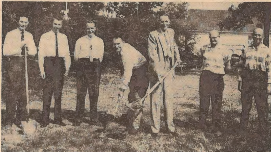
OAK CLIFF breaks ground for new building. Left to right: Hill, Goodman, Ibson, Bucella, Pastor Walker, Narrimore, and Woodward.
