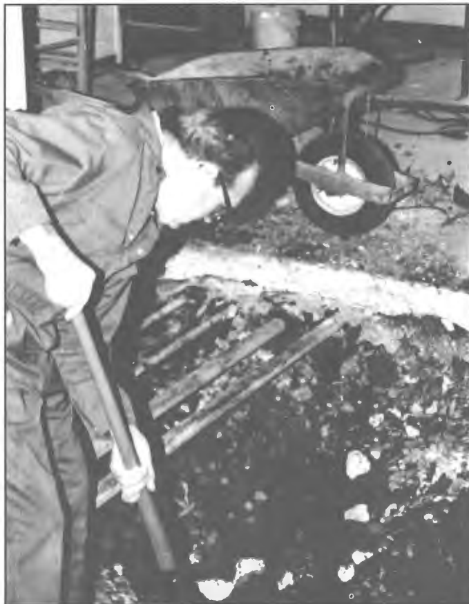
HOLIDAY CONSTRUCTION • The Christmas holidays provided a few days of needed renovation in Berry Bible Building. A new elevator was installed in the area between the classroom building and chapel.
