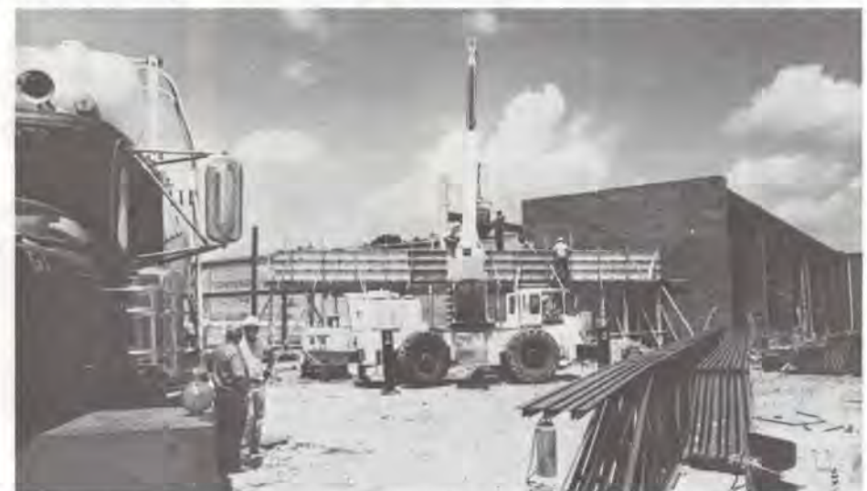
HPER BUILDING—A construction crew works on Ouachita's $4 million health, physical education and recreation complex. The project is part of the school's Centennial Advancement Campaign leading up to the 100 anniversary of the institution in 1986. Pickens-Bond Company of Little Rock is the primary contractor of the new structure, which, when completed in the spring of 1983, will adjoin Rockefeller Field House.
