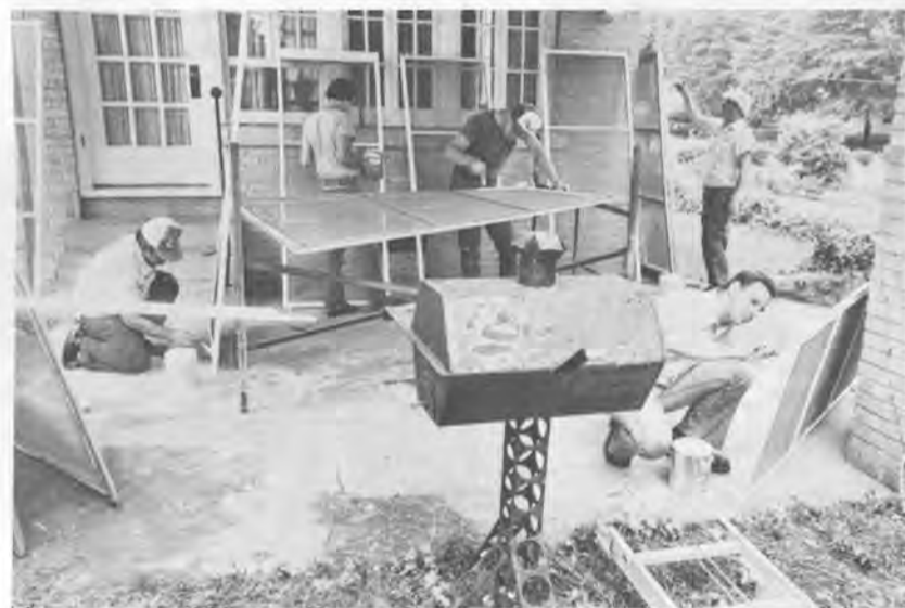
Workers spruce up Home Management House (L), install pitched roof on Moses-Provine.
