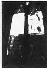
Shattered stained glass at Oklahoma City's First Baptist Church.
