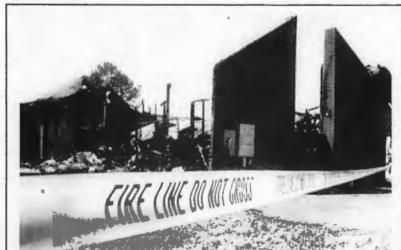
The main building of Remount Church in North Little Rock, including the 300-seat sanctuary, library and offices, burned early March 31 after being struck by lightning. The congregation is meeting in the church's education building. "We don't know why God allowed this to happen," said pastor Victor Coleman, "but He's still in charge and He promises to see us through any problem." Members plan to begin rebuilding this summer and complete it before Christmas.
