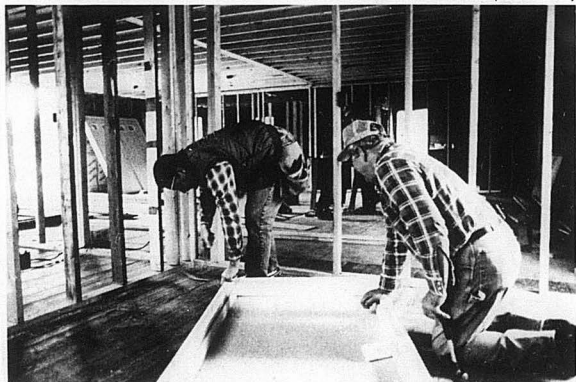
First Southern Church in Bryant is renovating a building for their mission at Ranche Acres near Alexander. A volunteer crew under the direction of Walter O'Neal has been working on the house, which was cut in two and moved to the church site. There the halves were separated and a new section added between them. The men from First Southern were joined Jan. 28 by a team of Baptist Men from Otter Creek First Church in Little Rock.
