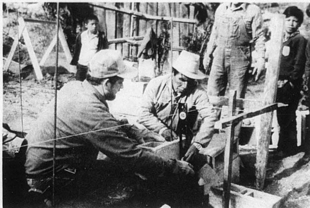
Keith Knupp (left) and a local Guatemala man work on a church foundation.
