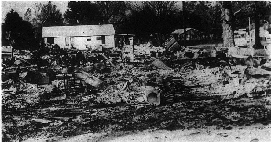
Leachville Second Church was destroyed by fire Nov. 14. Pastor Roger Haney is confident they can rebuild with God's help.
