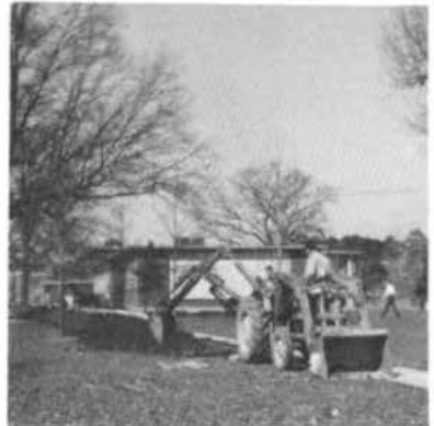
A Ouachita student looks on as the pipeline ditch is dug and preparations for the chapel begin.
