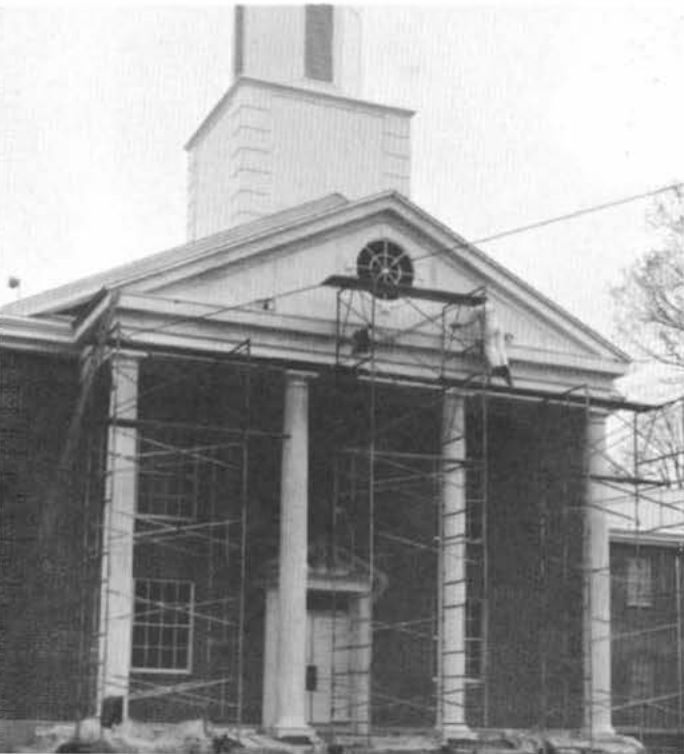
A workman puts the finishing touches on as he paints the front of the building.
