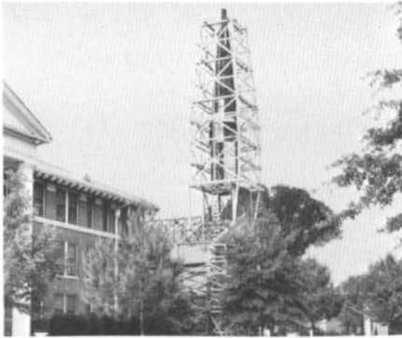
Scaffolding surrounds the steeple as preparations are made to cover it with aluminum.
